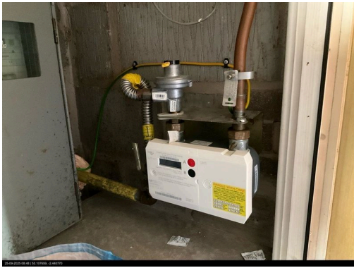
Photo of Gas Meter:
