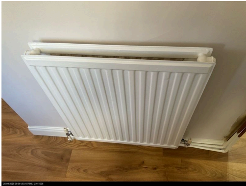
Photo of heating system:
