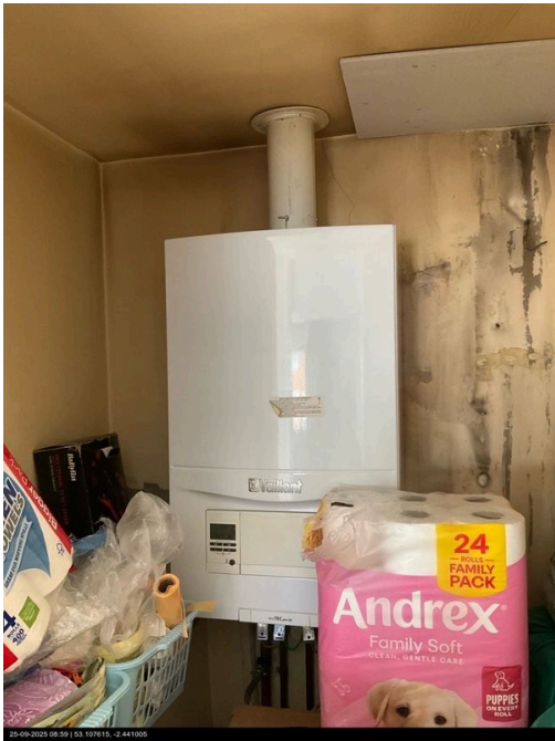
Photo of heating system:
