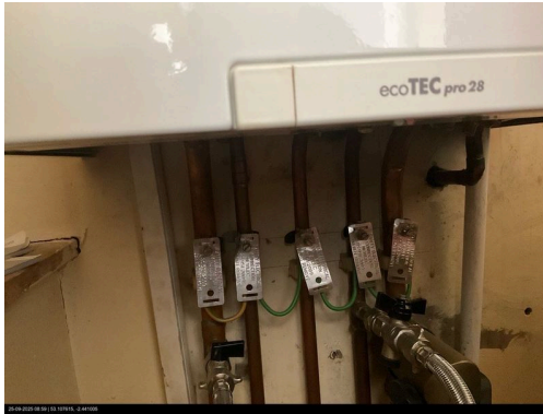
Photo of heating system:
