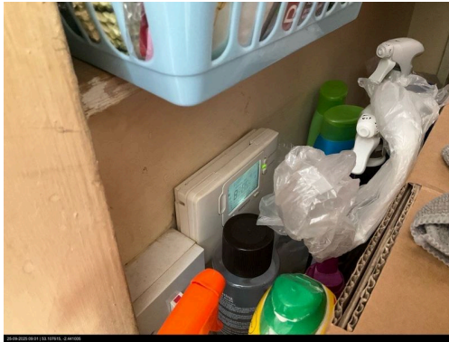
Photo of heating controls:
