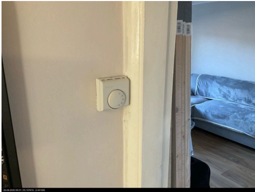
Photo of heating controls:
