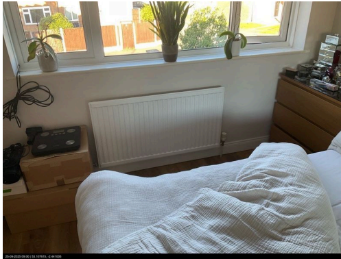
Photo of heating system:
