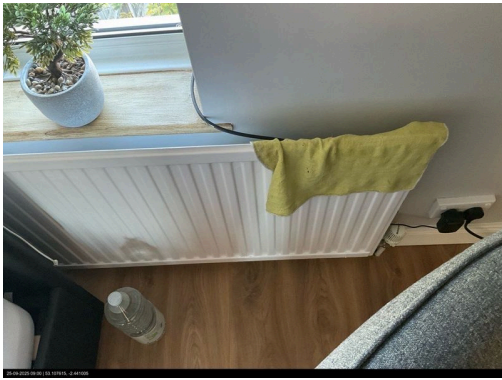
Photo of heating system:
