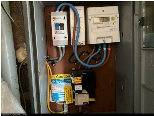
Photo of electricity meter:
