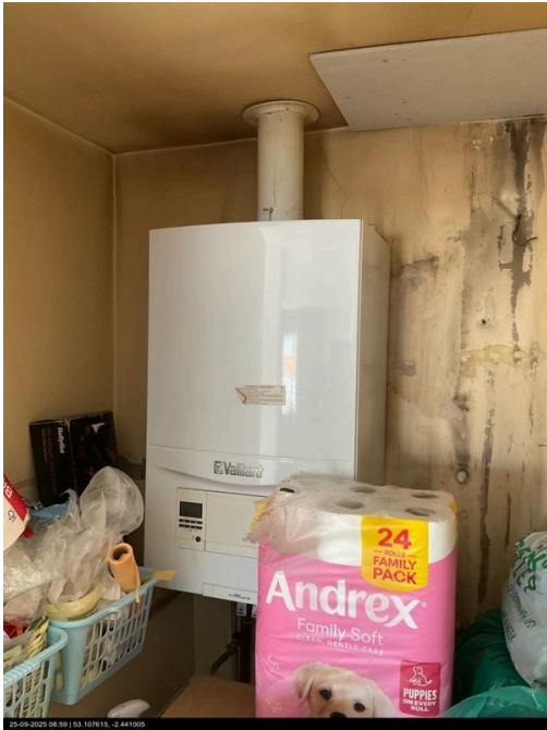
Photo of heating system:
