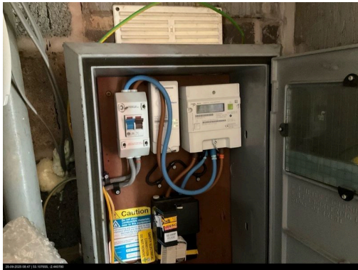
Photo of electricity meter:
