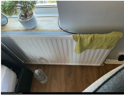
Photo of heating system:
