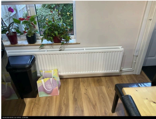
Photo of heating system:
